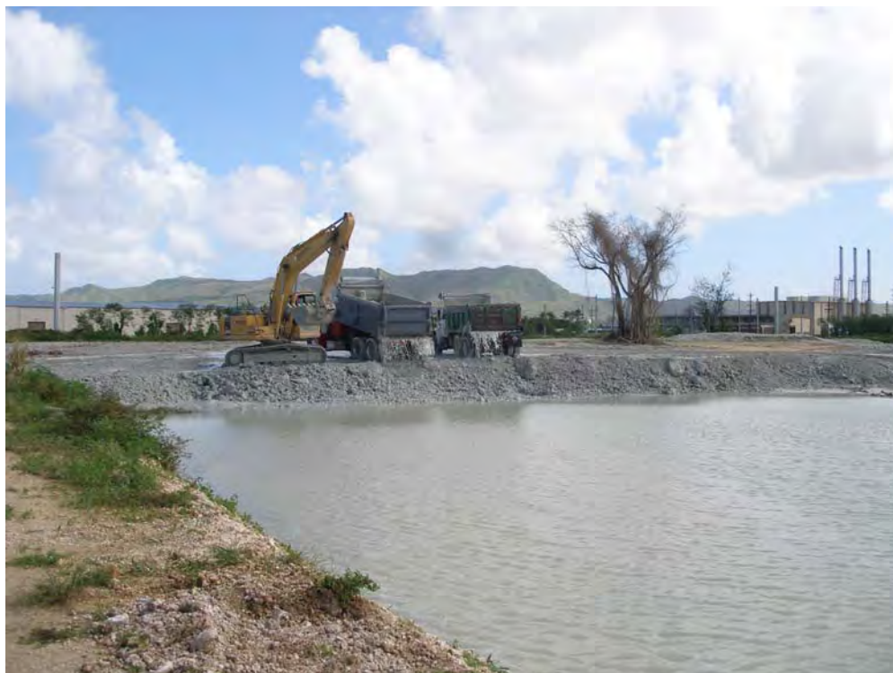
Figure 11. Existing conditions in 2007 at Field 5 Dewatering Facility, Cell 2, between Sumay and Marina Drives, Apra Harbor, Guam.
