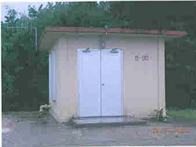
Booster Pump Station – Photo From UTS 2005
