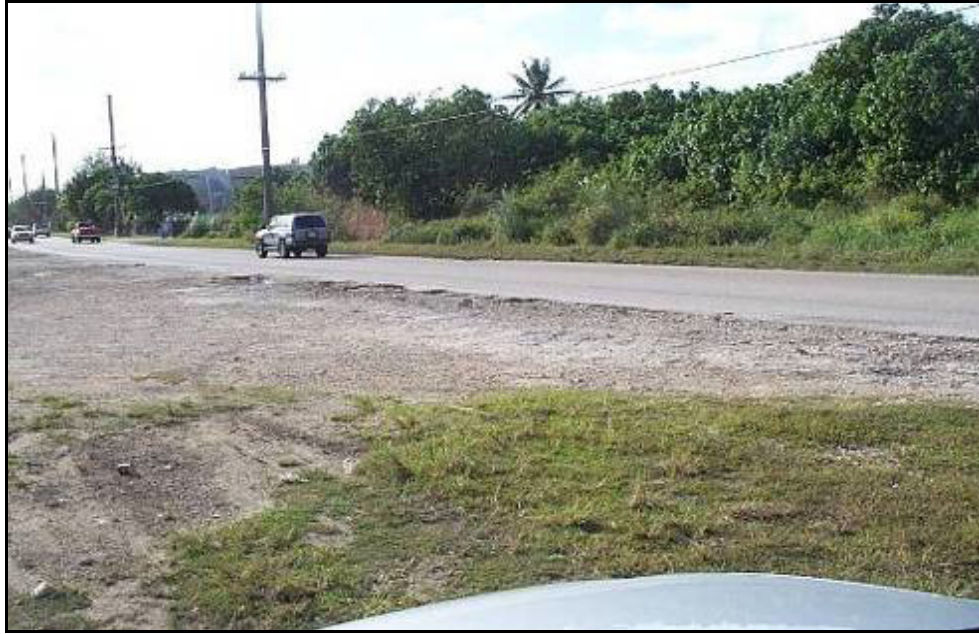
Figure 4.1-21. Route 27 Asphalt Damage
