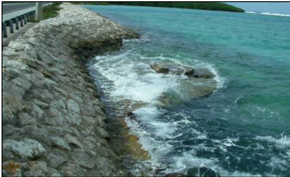
Figure 4.1-38. Coastal Erosion Protection along Route 11
