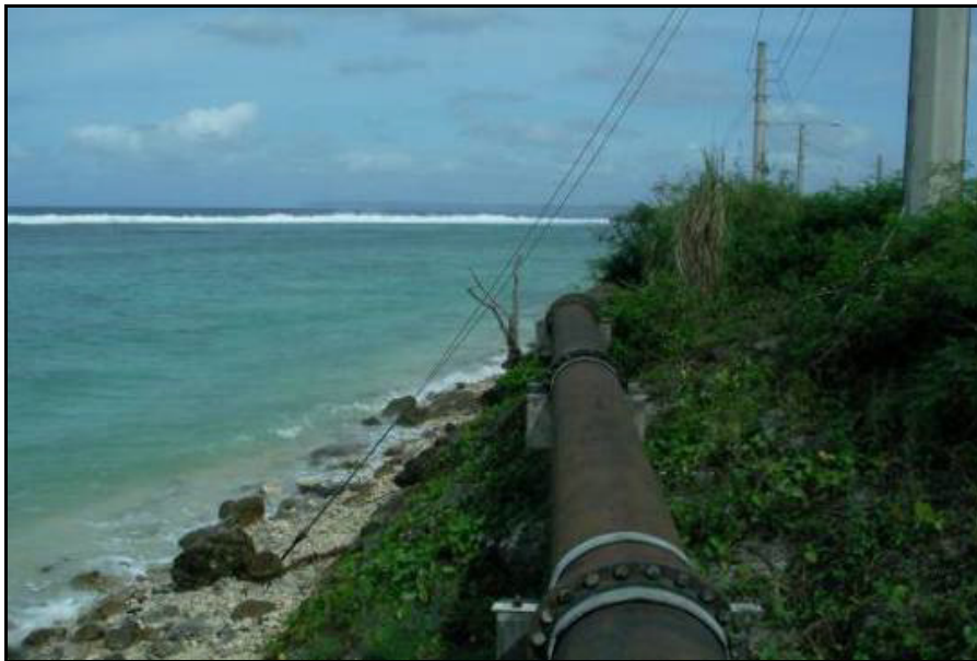
Figure 4.1-26. Coastal Erosion Protection along Route 1
